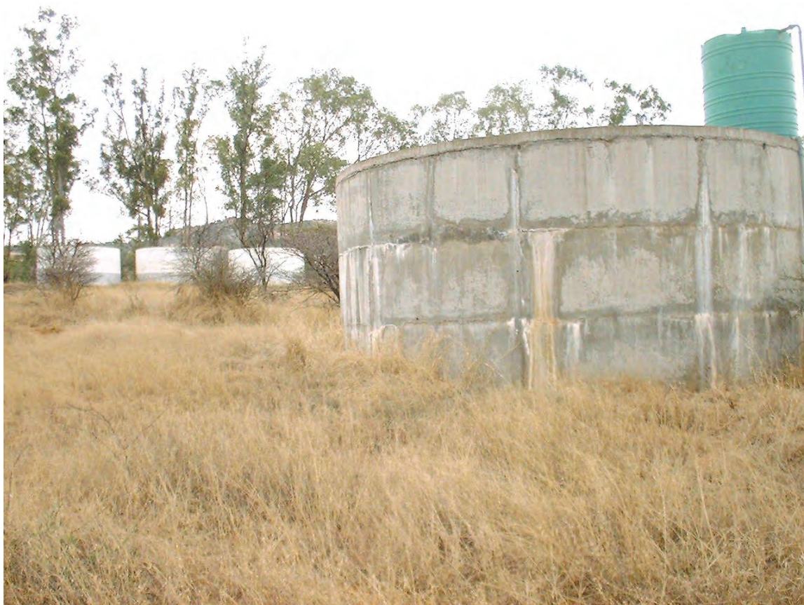
Figure 3. Turfloop Hatchery water supply header tank (foreground) and sand filter tanks (white, in background).
