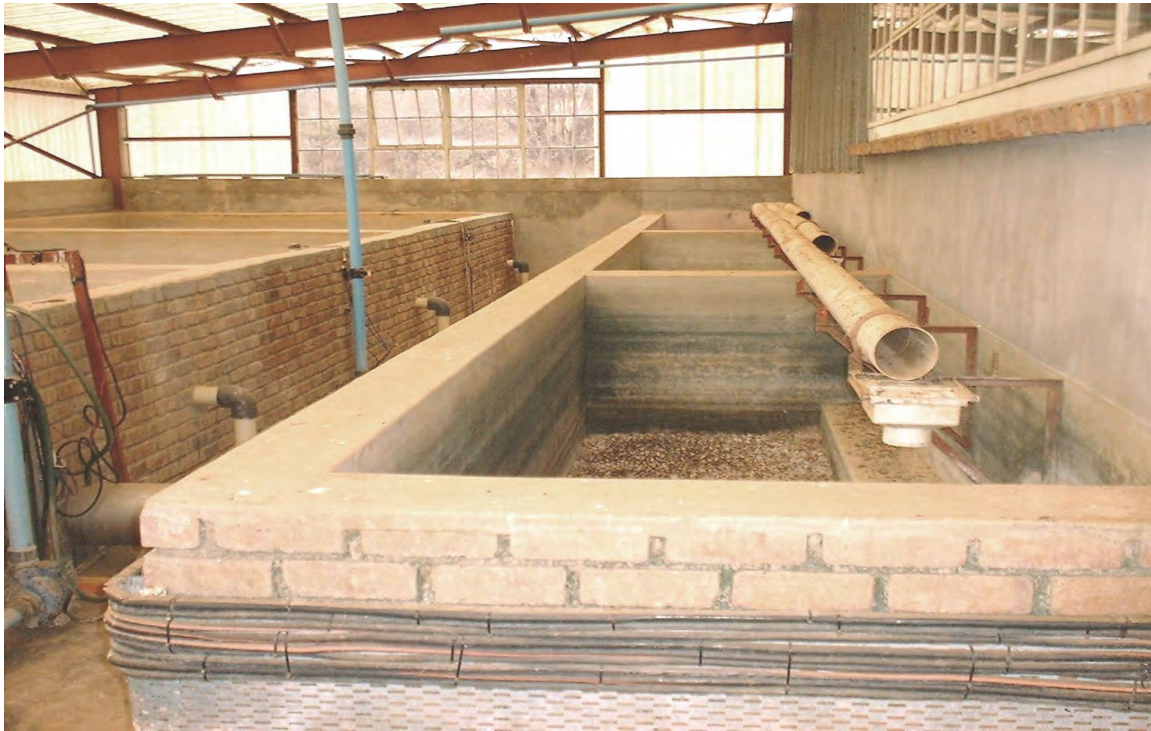
Figure 4. The indoor hatchery filter room. The large white pipe directs effluent water from the fish-tanks into the primary filter chamber which then overflows to the large secondary tanks to the left of the picture. The pumps, which draw water from these, are situated at the base of the blue pipes. The third pump is missing.
