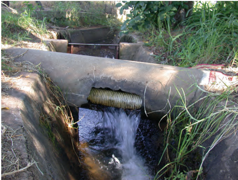
One of the many broken pipes at Lydenburg Hatchery.
