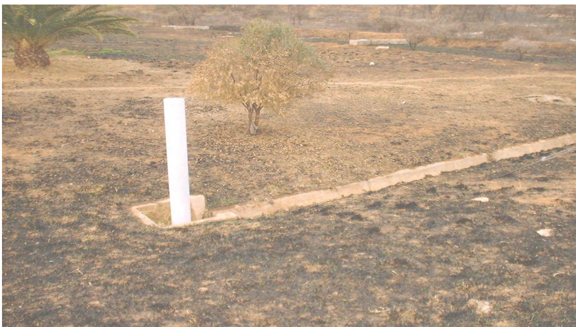
Figure 10. Pond outlet pipes are positioned outside the ponds as up-stand-pipes that are 'turned down' into the drainage canal for draining the pond. Some of these PVC pipes have been burnt and require replacement.
