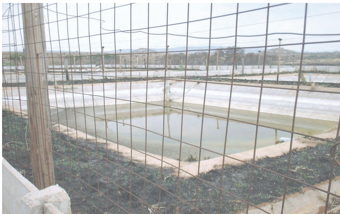
Figure 8. Concrete-lined ponds behind walls and mesh fences to exclude predators. All the ponds are either partially or completely empty (October 2006).
