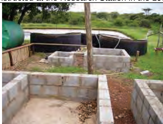
Figure 4: Incomplete fingerling system which has remained so for the last three years
