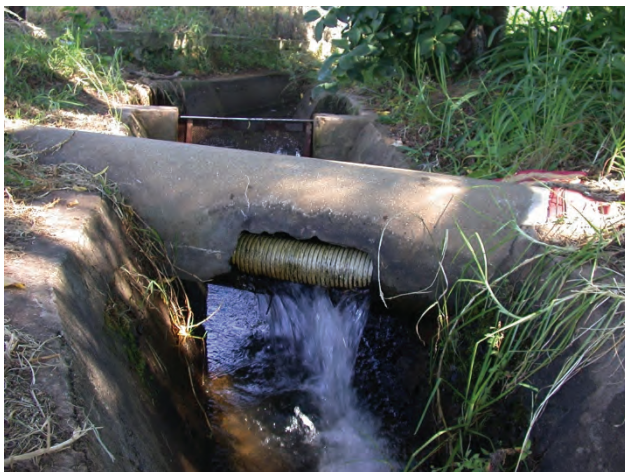
Figure 22. A broken pipe at Lydenburg Hatchery. The province will need to invest in infrastructure upgrading at this facility.
