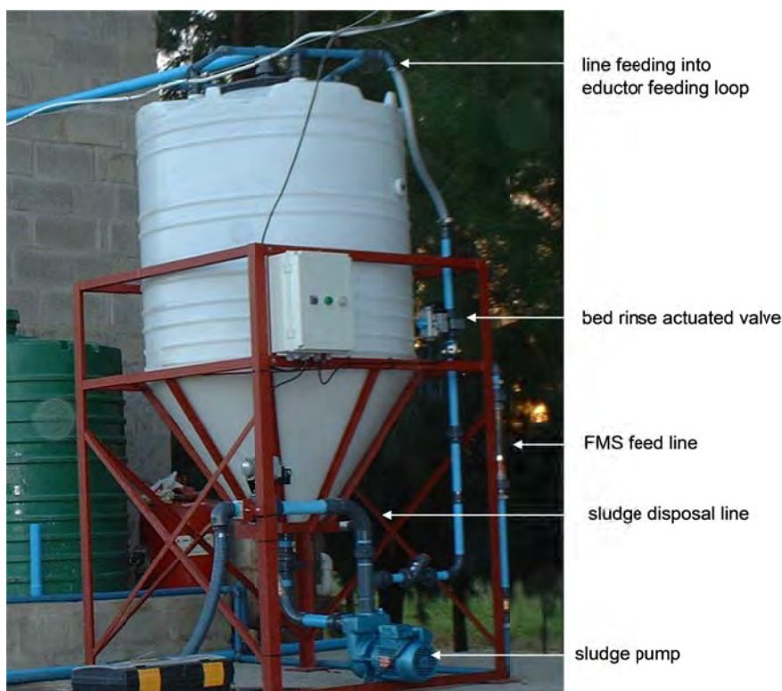
Figure 42: First FMF prototype installed on a grape farm near Piketberg to treat water from the Berg River.
