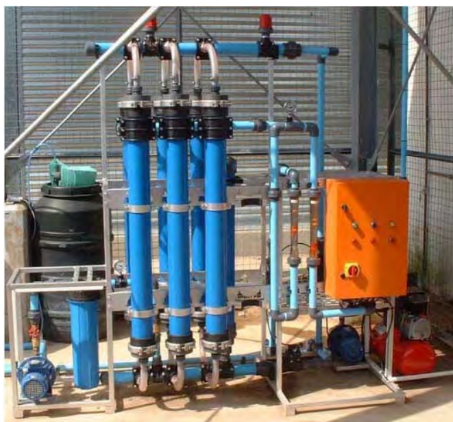
Figure 52: CUF plant operating on borehole water containing (6 mg/L) dissolved iron.
