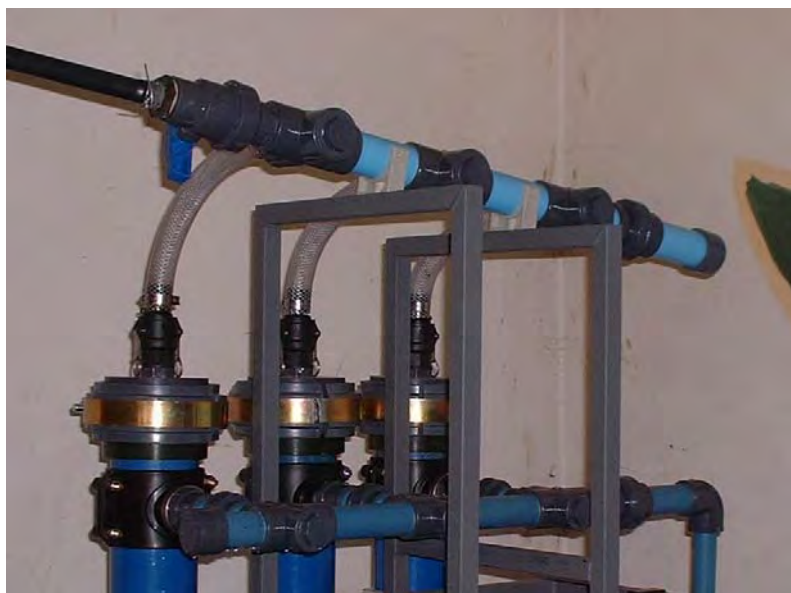
Figure 45: Top manifold with PVC cross-pieces and flexible hose connection to the modules.
