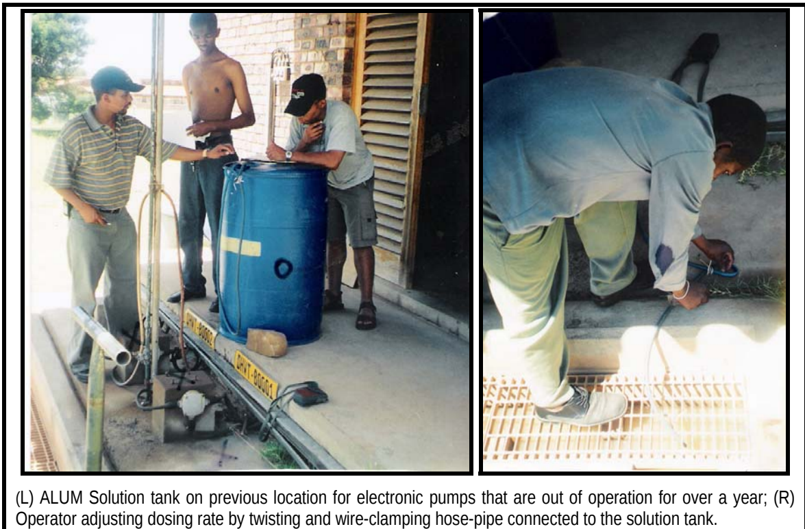
Figure 2-10: Gravity chemical dosing system in Cofimvaba – Eastern Cape
