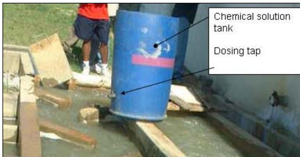
Figure 2-6: Drip chemical dosing system - Ashton, Western Cape
