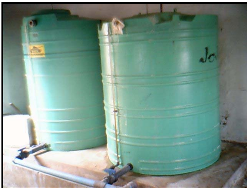
Figure 2-9: Gravity chemical dosing tanks in Bonnievale – Western Cape
