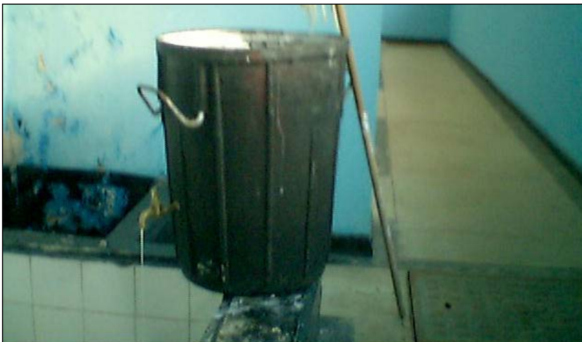
Figure 2-11: Emergency gravity chemical dosing system-Fort Beaufort, Eastern Cape
