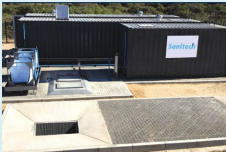
Figure 16: Image of the Santech modular, portable WWTW (taken from Sanitech (undated))
