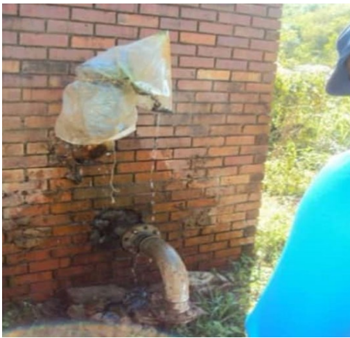
Figure 2.2: Damaged and leaking pipe in a rural community in South Africa (Source: Mothetha et al., 2013)
