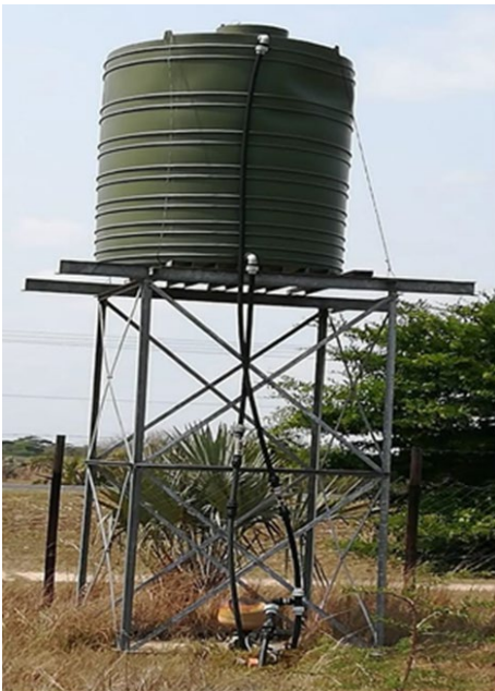
Figure 3.1: An electric pump used for drawing underground water into a water tank in Ndlondlweni, Umhlabuyalingana Local Municipality
