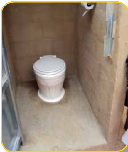
Pour flush toilets selected for conversion to low flush systems
