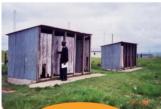
Toilets with broken down doors and unsteady structures
