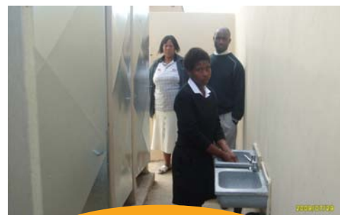
Inside toilet block with hand wash basin and new doors for toilets
