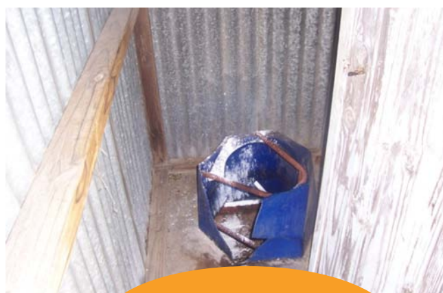
Toilet with broken pedestal
