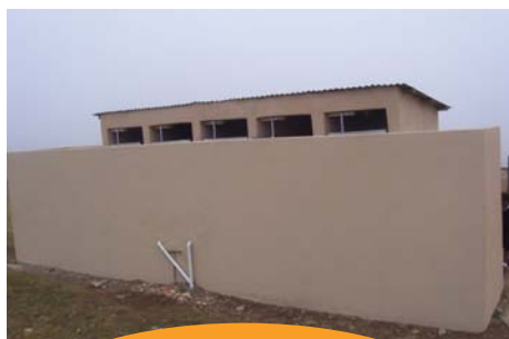
Pipes for water supply of the hand-wash basins. Girls toilet block re-plastered and painted
