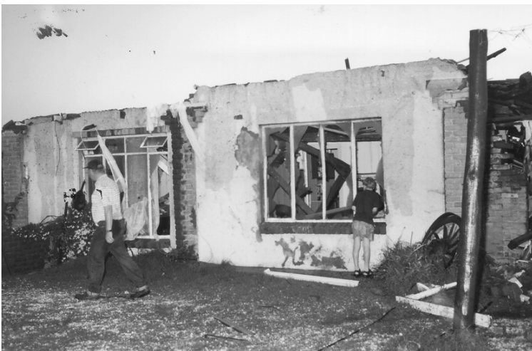
Figure 6 Damage to a farmhouse (Goliger and Van Wyk, 1999)
