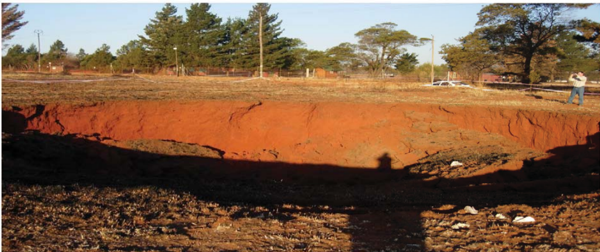
(c) Sinkhole in Bapsfontein, further developed over a period of ten years (City of Ekurhuleni, © JL van Rooy 2017).
