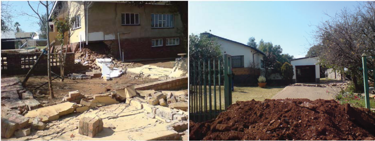
(a) Damage to house due to sinkhole (left) and to adjacent property (right) in City of Tshwane in 2012
