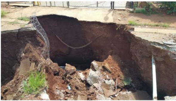
(a) Sinkhole in Khutsong, 10 m diameter (24 January 2018).
