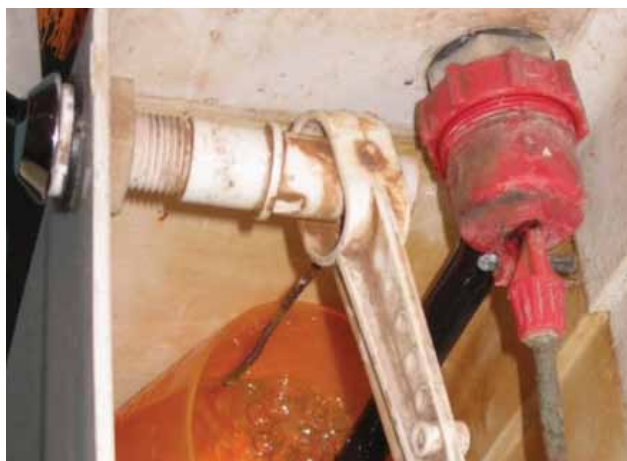
Figure 1: Cistern leaking 1ℓ every 23 seconds
