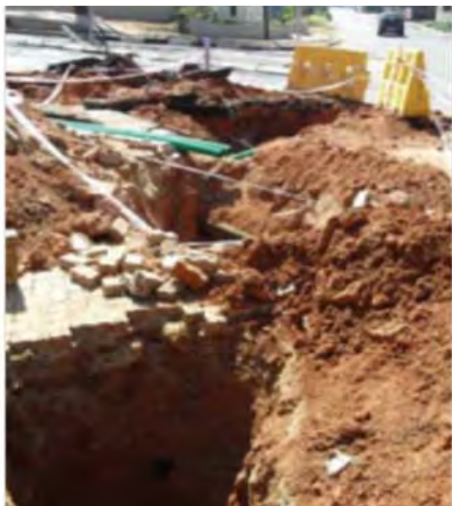
Figure 2: Extensive excavations undertaken in the Sandton area to expose and trace the position of a leak from an underground pipe
