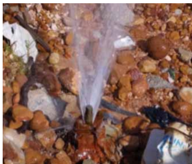
Figure 3: Leaking valve located on bulk supply pipeline
