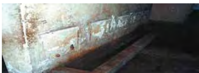
Figure 5: (Before) Missing basins in hostel due to vandalism and theft
