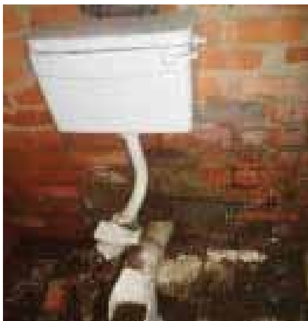
Figure 3: Vandalised toilet soon after installation
