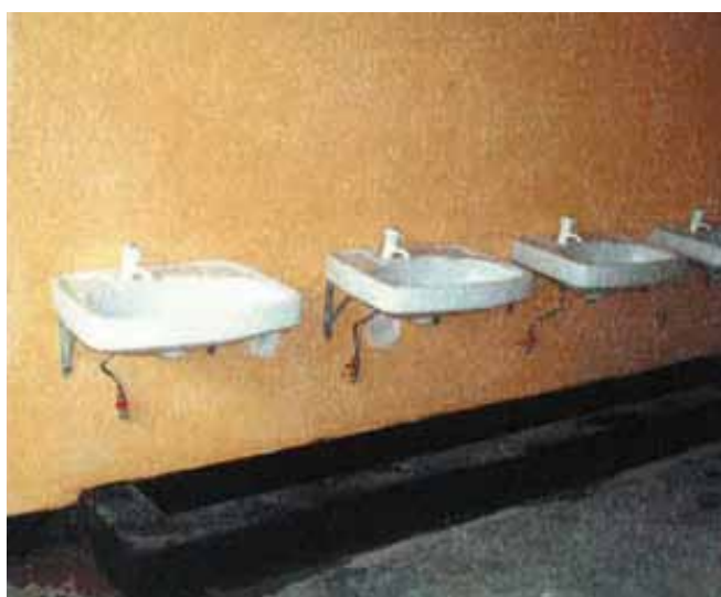
Figure 6: Basins with water efficient faucet installed
