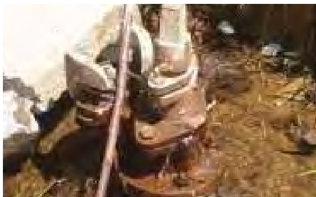
Figure 2: Leaking network valve
