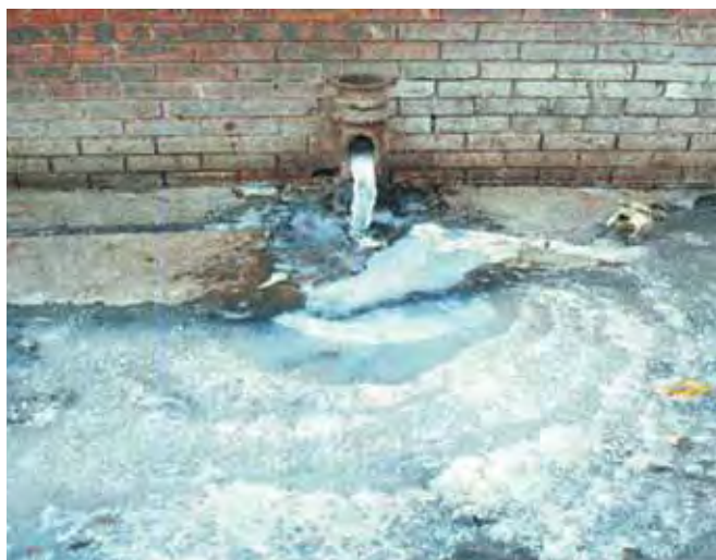
Figure 2: Madala Hostel effluent flowing directly on to property
