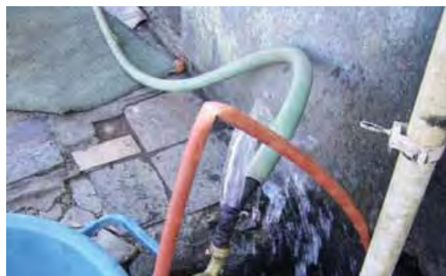
Figure 1: Leaking plumbing fixture
