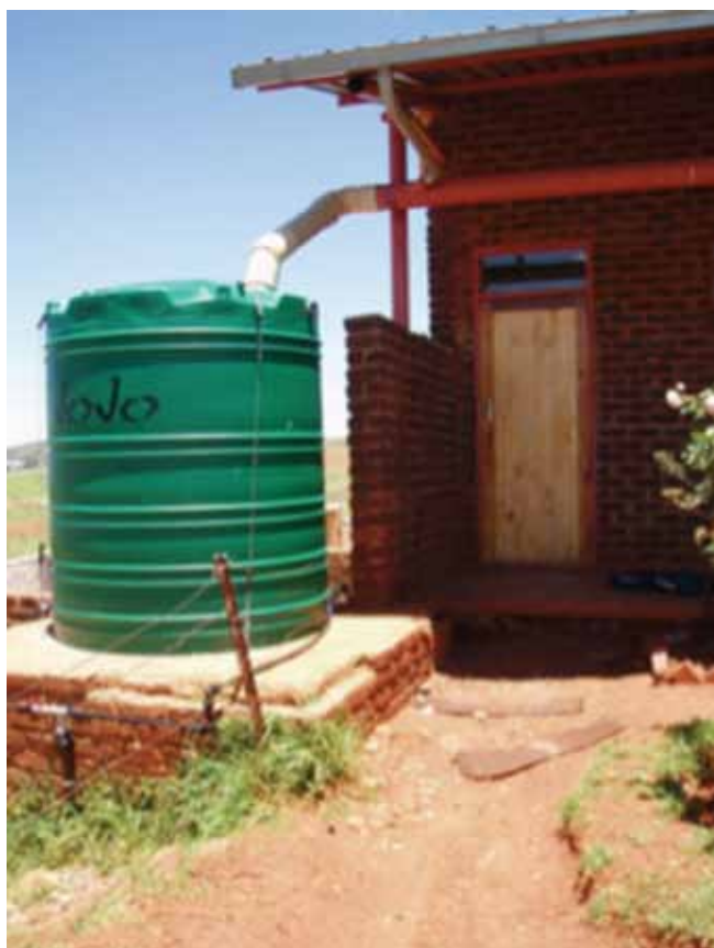
Figure 4: The borehole supply is now used for drinking and the rainwater (harvesting tanks installed through project) is used for flushing the toilets. If there is a shortage of rainwater, then borehole water can be diverted to flush toilets
