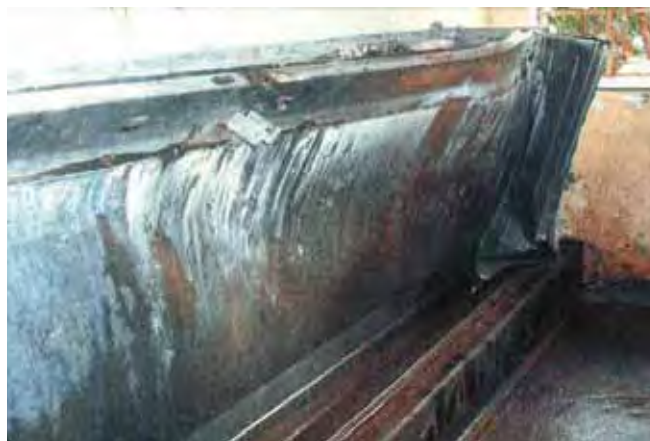
Figure 3: (Before) Leaking automatic flushing urinal
