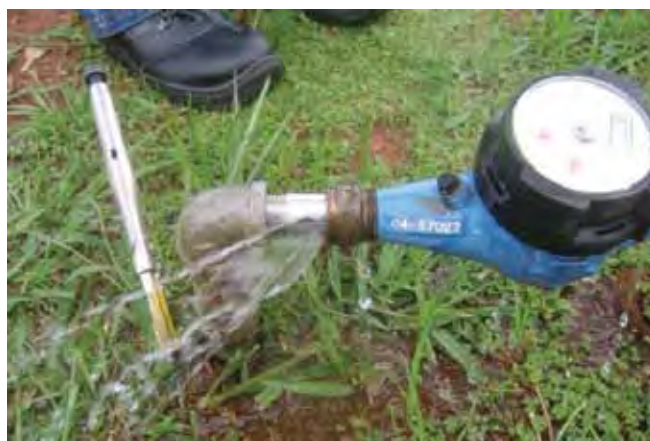
Figure 3: Leaks observed at meter
