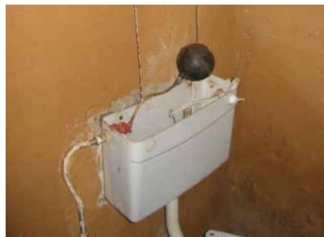
Figure 2: No Operating Float valve to stop the cistern from over-filling
