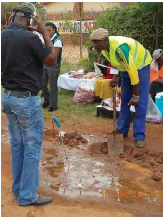
Figure 3: Underground leak identified by ALC team
