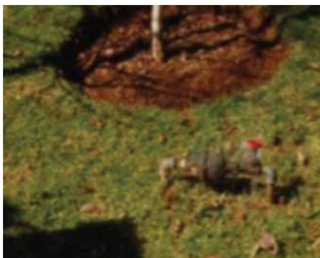
Figure 3: Leaking municipal connection
