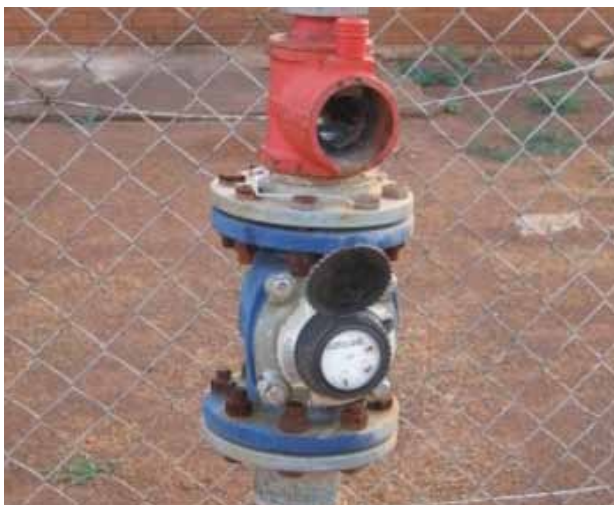
Figure 1: Incorrectly placed meter
