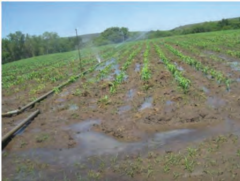
Plate 4.10: Leaking pipes cause water logging in portions of the scheme. Risers on this lateral line are of different heights affecting water distribution
