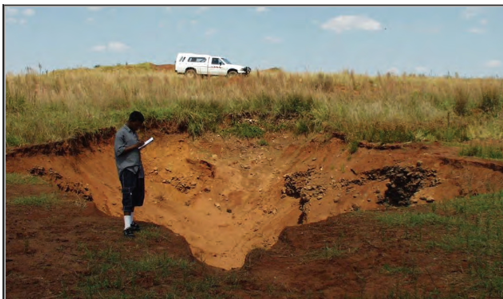
Figure 10.4: One of the sinkholes in the dry streambed of the Tweelopiespruit West immediately downstream from Tarlton. These sinkholes were formed due to the increased flow in the stream and also due to the removal of the peat beds in this stream (run-off attenuation properties of peat lands and associated reed beds), allowing storm water to flow further downstream before recharging into the dolomitic aquifer (photo: W.G. Krige 31/03/2002).
