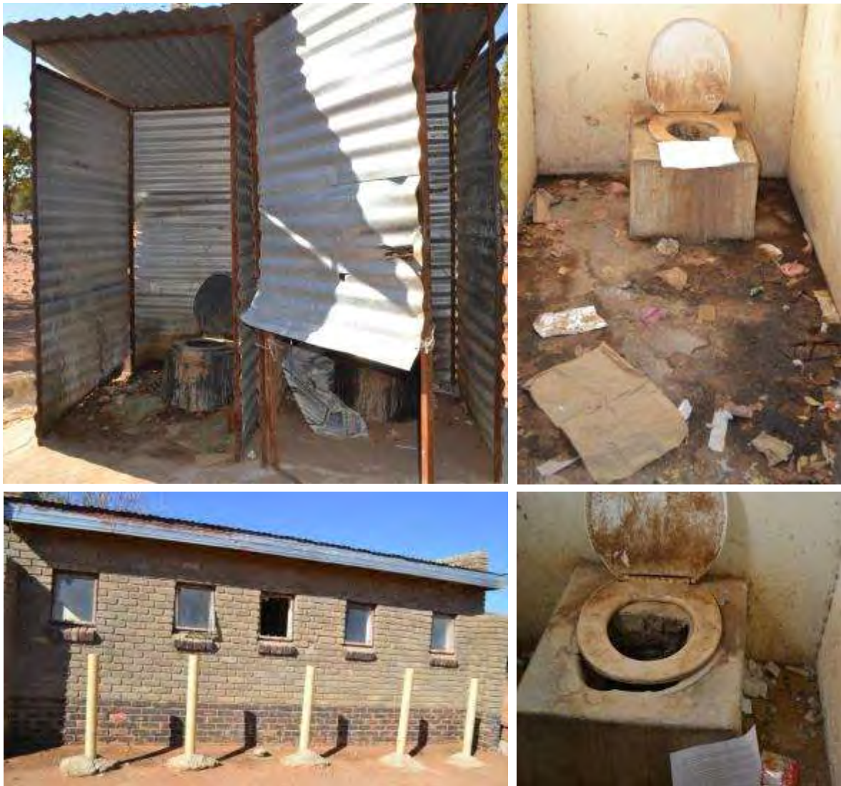
Figure 11 Toilets without doors, vents pipes without covers and inadequate pedestals at Tshianane
