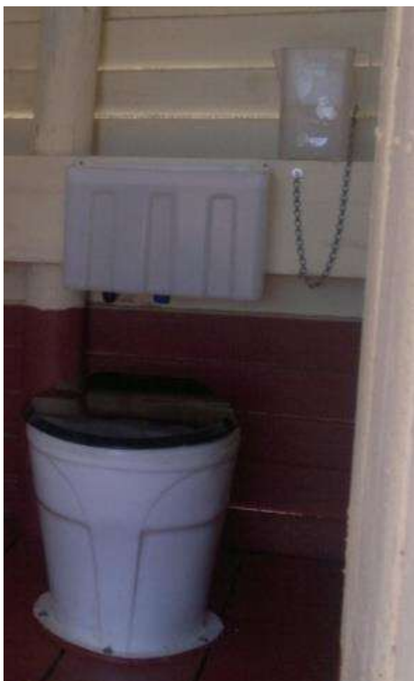
Figure 47 Pour flush design used at schools in Limpopo with water dipped from a cistern kept at a constant level
