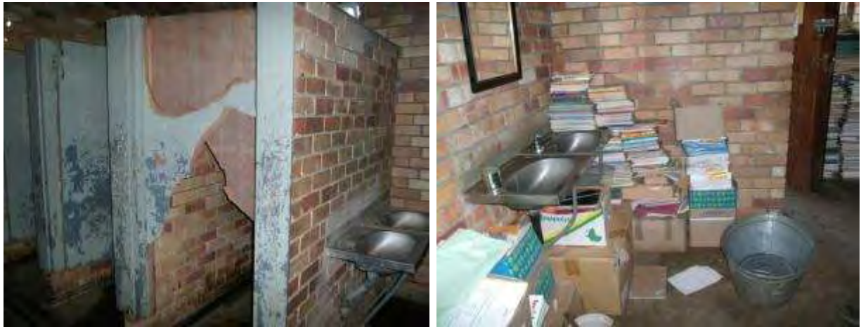
Figure 9 Broken doors and missing taps at S W Mbanga Junior Secondary School
