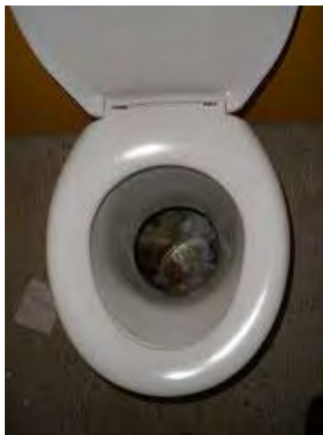
Figure 50 Enviro Loo toilet block (left) showing vent pipe and black collection chamber covers and pedestal (right)
