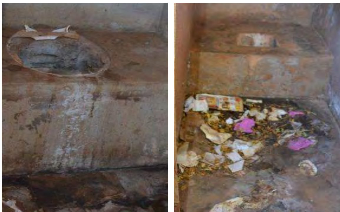
Figure 21 Toilets with broken or missing seats at Humbelani
