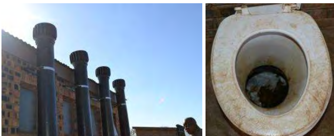
Figure 19 Vent pipes and full toilets at Jaji Secondary School
