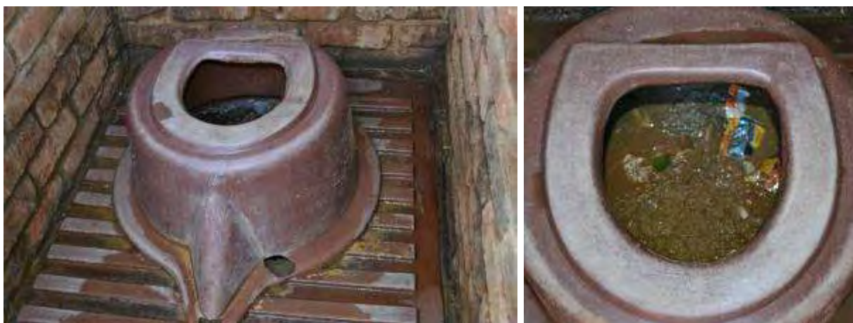
Figure 20 Full pit latrines at Pholoahlaba
