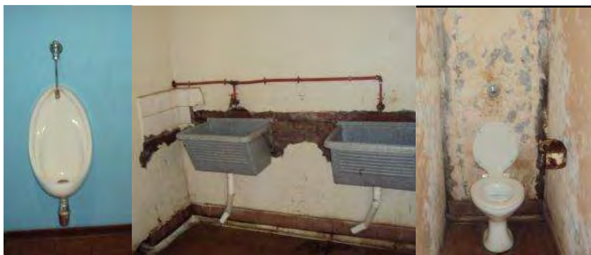
Figure 15 Male staff toilets (left) and sinks and toilets for learners (centre and right) at Georgetown High School
