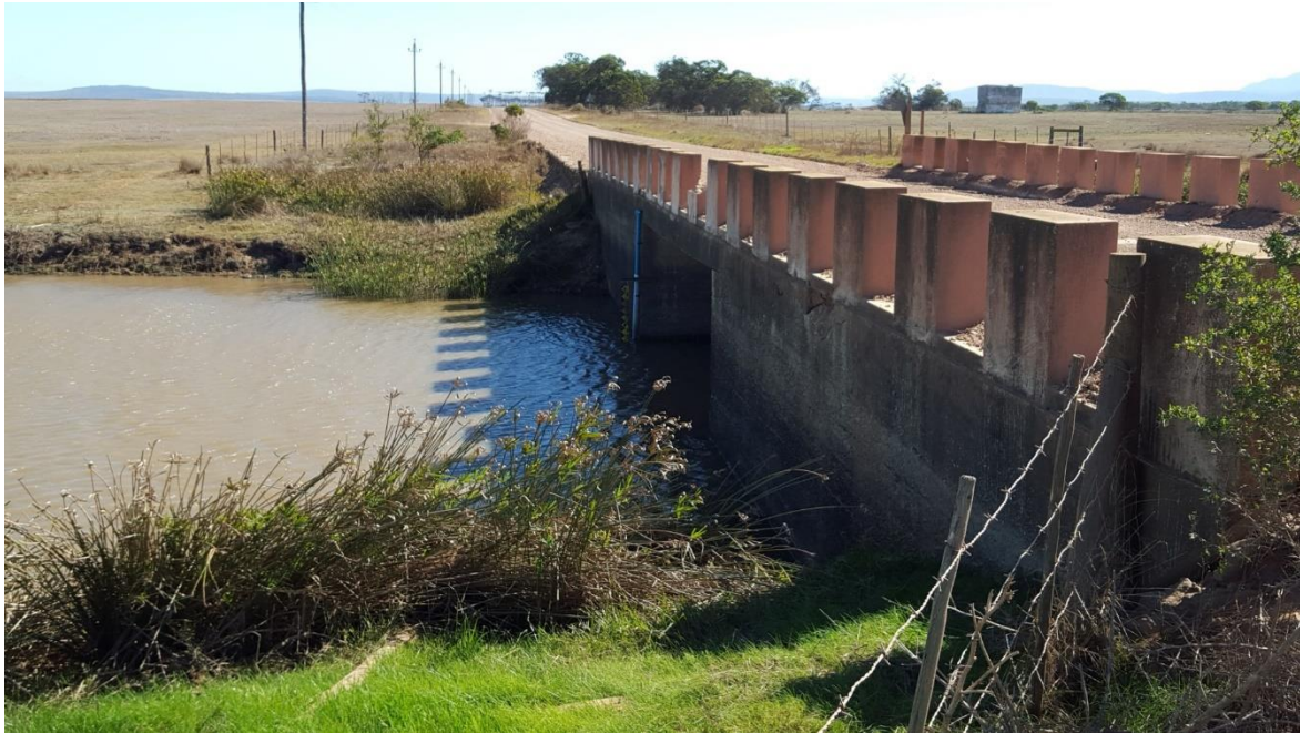
(a) Stilling well (blue PVC) with data logger in the Voëlvlei River at the Elim-Struis Bay road bridge
