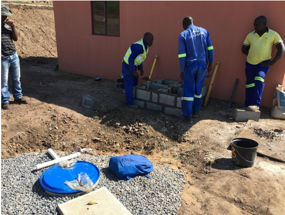
Figure 11: A greywater recycling system under construction in the foreground. In the background a stand is being constructed for a rainwater harvesting tank.
