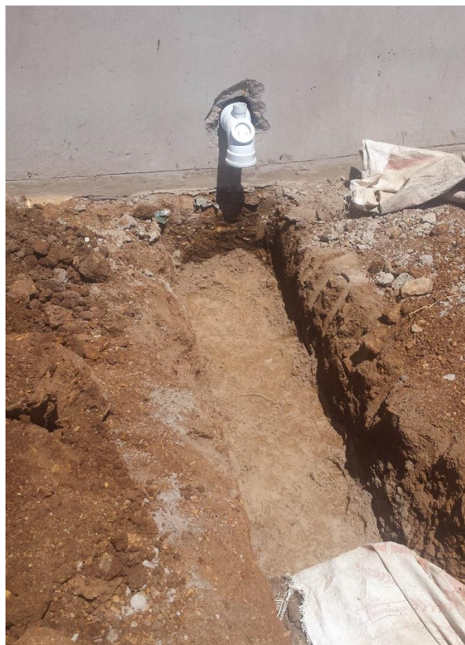
Figure 7: Bedding and blanketing material has had to be imported from commercial sources to protect the pipes.
