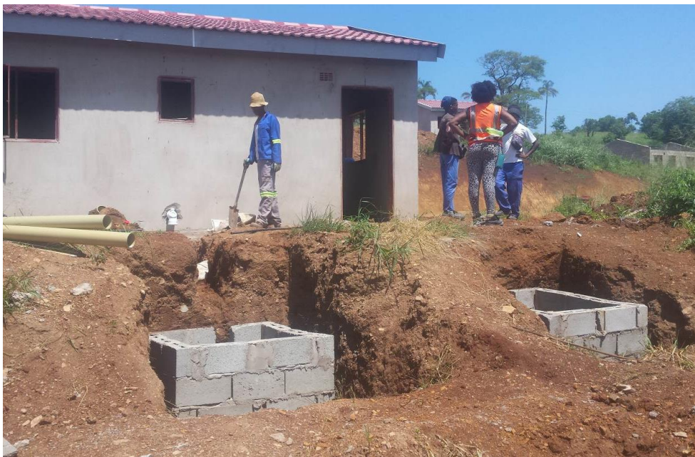
Figure 10: A view of leach pits under construction at one of the Oakford houses.
