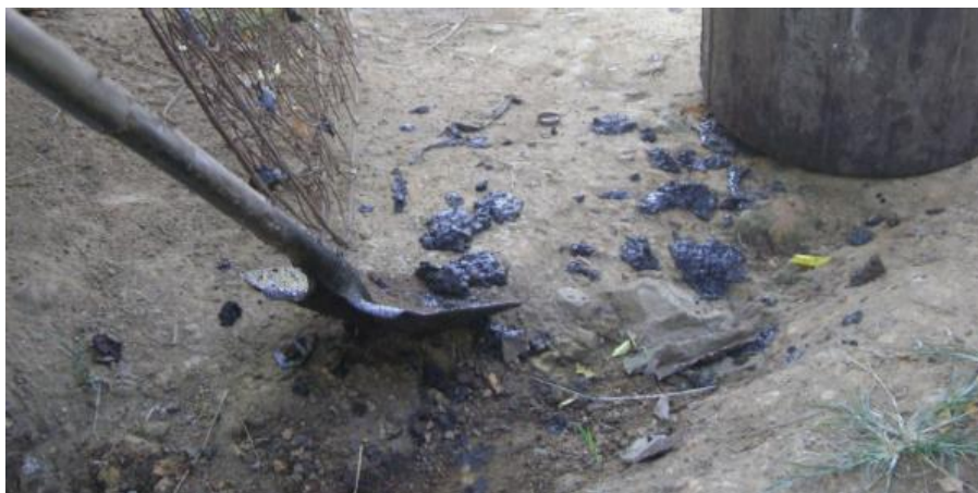
Figure 34: In some instances, workers attempted to remove sludge that had fallen on the ground. They did not however have any equipment for sanitising the contaminated area.
