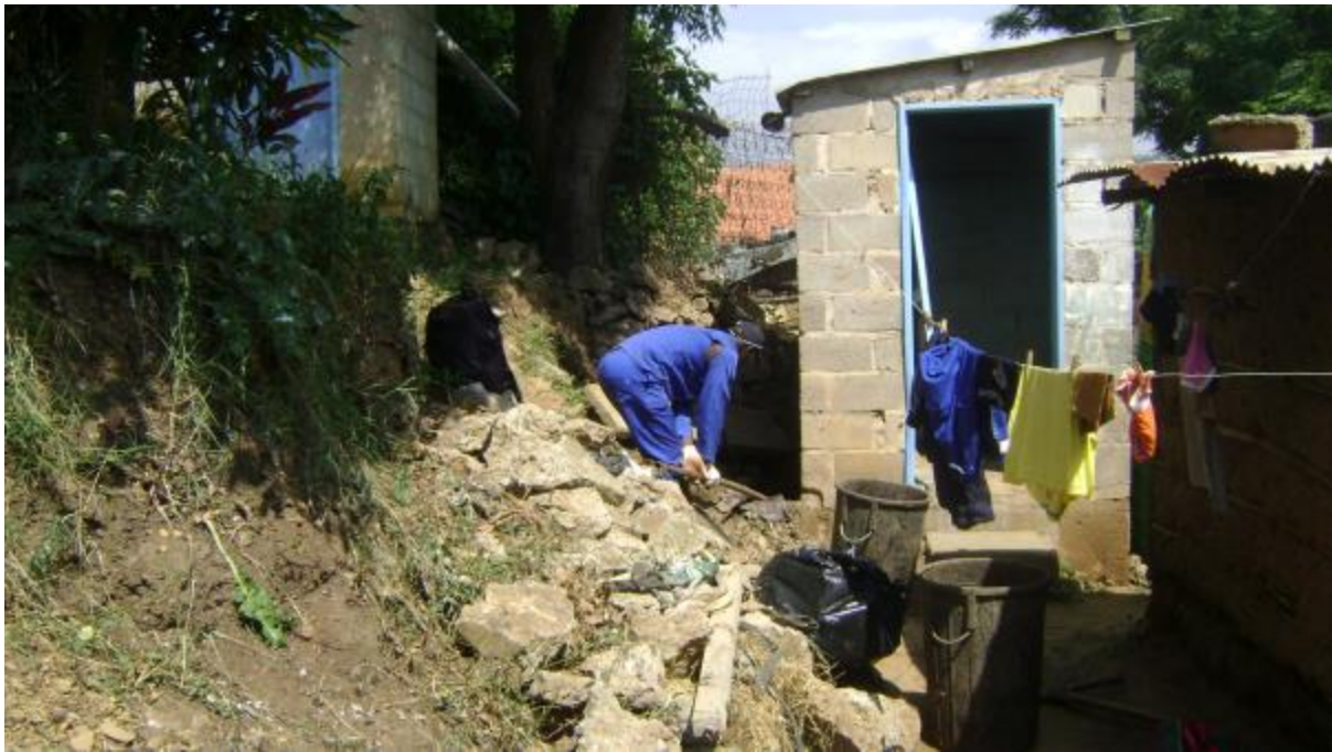
Figure 16: Pit emptiers working in cramped conditions placed their bins directly under washing drying on a line at this home.
