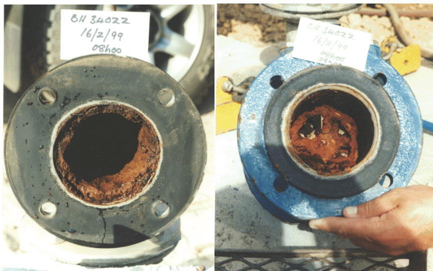
Figure 1: Clogging of a production borehole pipeline (left) and flow meter (right) as a result of the iron-rich groundwater experienced at the Atlantis Aquifer (More Water, 2001)
