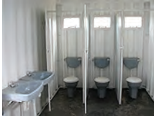
Figure 11: Internal view of the AB container
