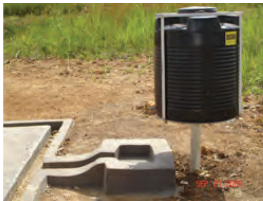
Figure 7: View of external hand washing post
