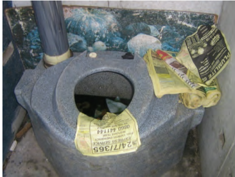
Figure 3: Condition of container toilets
