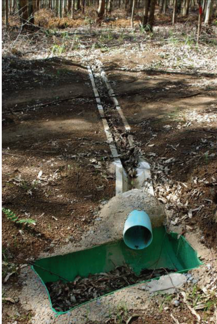
Figure 3.16. Water flowing within the gutter is directed into a stilling well. These were constructed from 210 L plastic drums that were cut in half lengthways.
