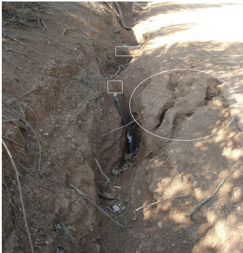
Figure 4.22. Severe gullying along the road verge at the section of the hillslope leading to the cut and fill embankment.
