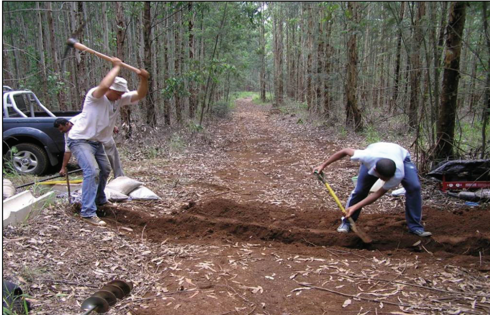
Figure 3.13. A trench of was dug across the road for installation of the concrete gutters.
