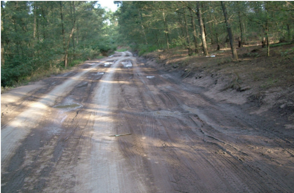
Figure 6.2. Road segment in moderate state of degradation.
