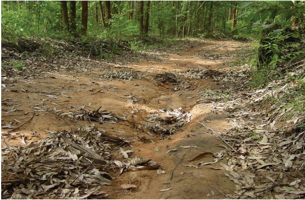
Figure 6.3. Road segment in an advanced state of degradation.
