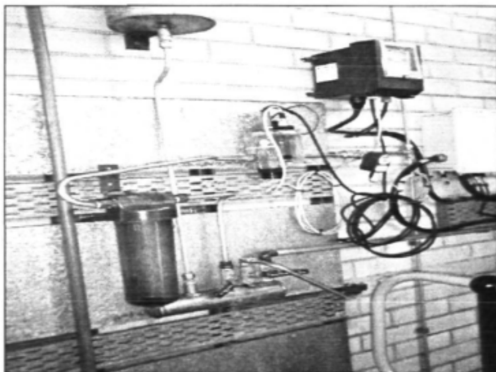
Figure 1.8 : On-line pH meter and Chlorometer at the exit of the reservoir
