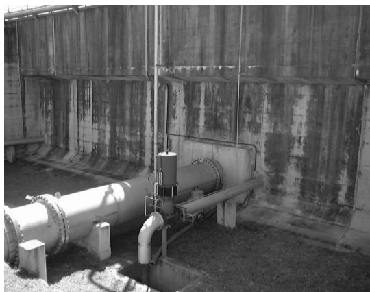
Figure 3.1: View of the ozone contactor, showing the static mixer at the inlet.
