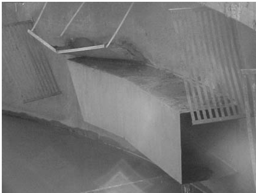
Figure 5.2: View of the peripheral feed inlet to the clarifier
