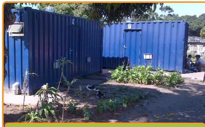
Photograph of community ablution blocks connected to ABRs in the Frasers settlement. Photo by Bjoern Pietruschka (2014).
